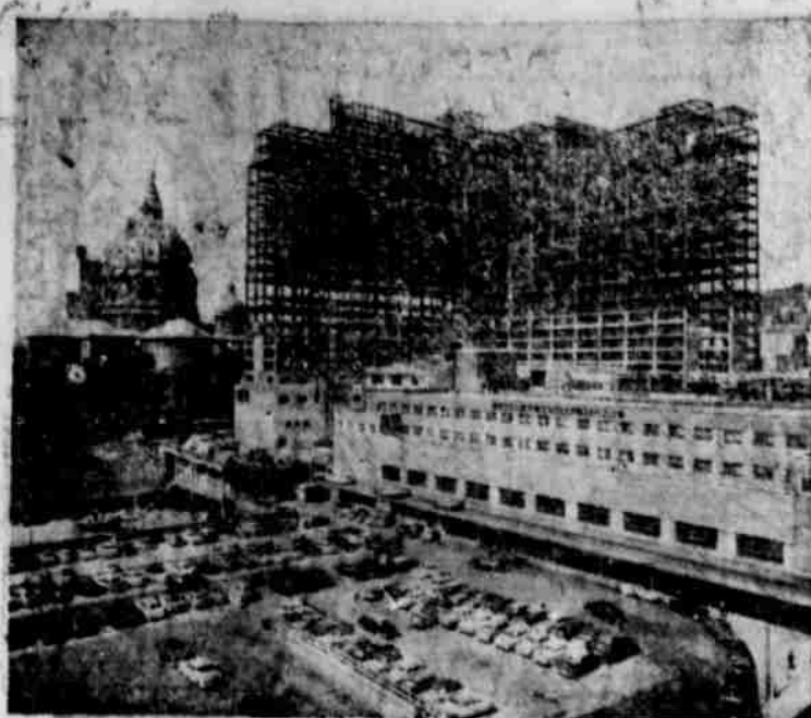
THE new "Queen Elizabeth" Hotel, a 21-story structure which will be opened in 1958, is taking shape on Montreal's "Place Ville-Marie." With more than 1,200 guest rooms, the "Queen Elizabeth's" public rooms will be capable of accommodating 2,500 persons at banquets and more than 4,000 at meetings.
