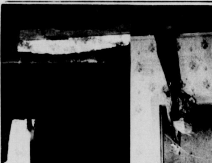
EXPLOSION: A gas explosion 2 miles West of Wheeler Monday evening resulted in injury to Mose Thompson. The explosion ripped the doors and windows from the house and left the front and rear walls pushed out from the foundation approximately four feet. The picture above shows the front wall of the house; the left of the picture shows where the front door and facing were torn from the house and light can be seen between the ceiling and wall. The picture on the right shows a pair of overalls suspended between the wall and the roof.
