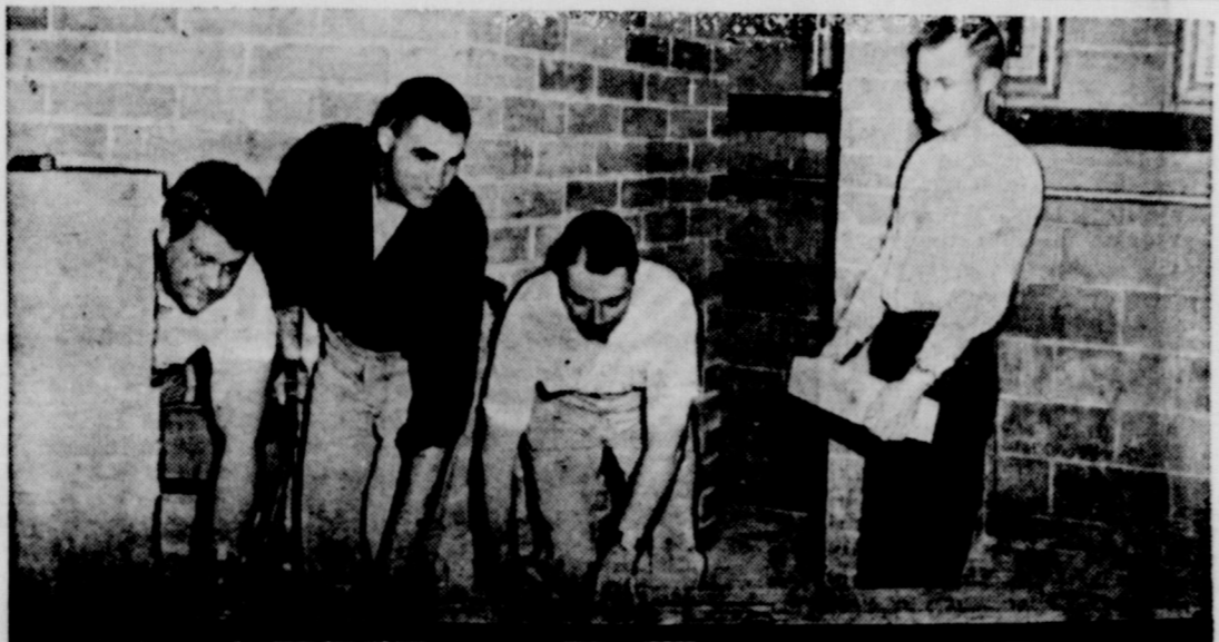
JAYCEE SHELTER project, part of the organization's nationwide "Operation Survival," takes concrete form as Blue Earth, Minn., Jaycees construct a 4-person fallout shelter in the city hall basement. This is one of a variety of permanent or temporary display shelters built by Jaycees in cooperation with civil defense in communities across the nation. Each of the 2,000 Jaycee chapters in the United States is being encouraged to participate in the program to stir public interest in fallout shelter construction in every community across the Nation. (Fairmont, Minn., Sentinel Photo)
