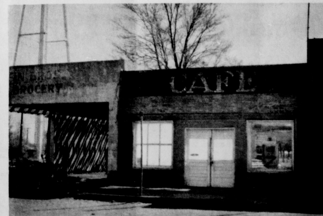
DOWN THEY COME: This is just one of the many improvements which have been started in Wheeler. These two buildings are being torn down to make way for a new modern Mobil Station. The razing of the buildings was begun Thursday. The widening of Shamrock street is being brought to a close with the paving nearly completed. The building of four new homes in Wheeler and the remodeling of one is under way. It has been reported that construction on a new motel will get underway soon. All this goes to prove that someone has a lot of faith in our community.
