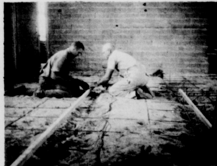
REMODELING: George Gandy and Mike Gandy are shown working on the gym floor where the stage used to be. The bleachers have been removed and a concrete floor has been run. The workmen are removing the light fixtures and will repair the ceiling and install the new fixtures. This work is under contract with Dorsie Hutchison.
