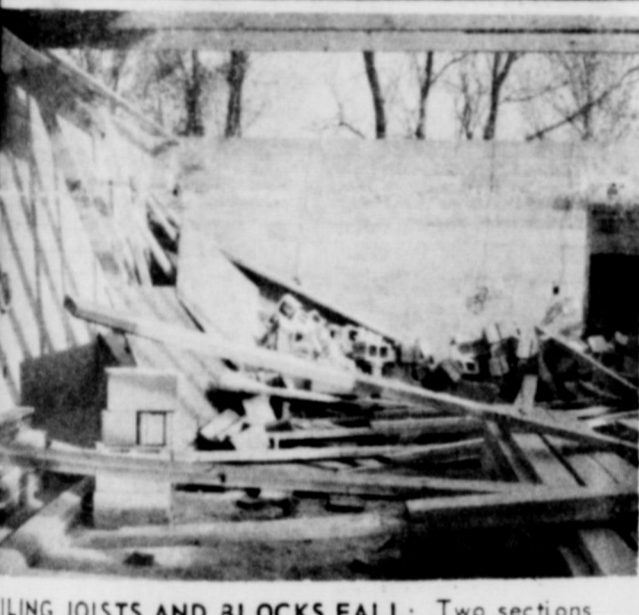
CEILING JOISTS AND BLOCKS FALL: Two sections of the roof fell on the City Offices and Fire Department meeting hall Tuesday afternoon when it was overloaded with blocks. This picture shows the back part of the building. One workman rode the scaffold to the floor and received only scratches.
