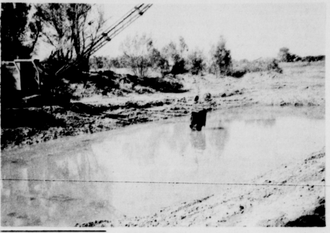
SEEP POND: This seep pond is being constructed on the Wallace Fields ranch west of Shamrock. This pond will not only furnish additional livestock water, but will be useful as a source of water for wildlife as well.
