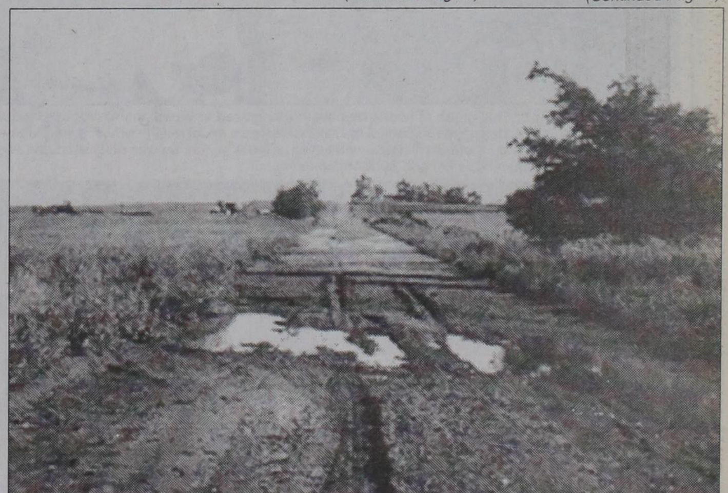
COUNTY ROAD 26: This is one of the pictures submitted by a group of Wheeler county citizens, who met with the county commissioners at their regular meeting Monday to complain about the condition of county roads. This picture shows the lack of ditches to drain the roads.
