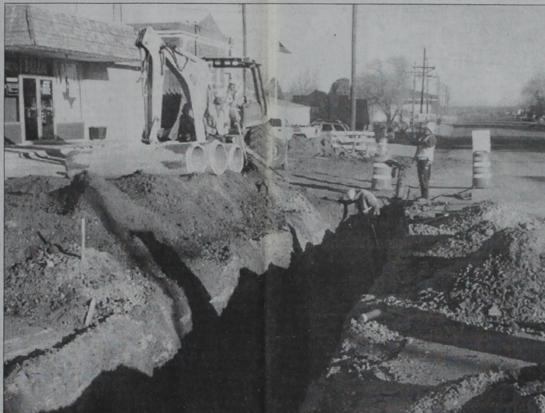
Workmen are shown here laying a waterline in front of Kim's Country Kitchen. This is only part of the work being done on Highways 83 and 152 in Wheeler.
