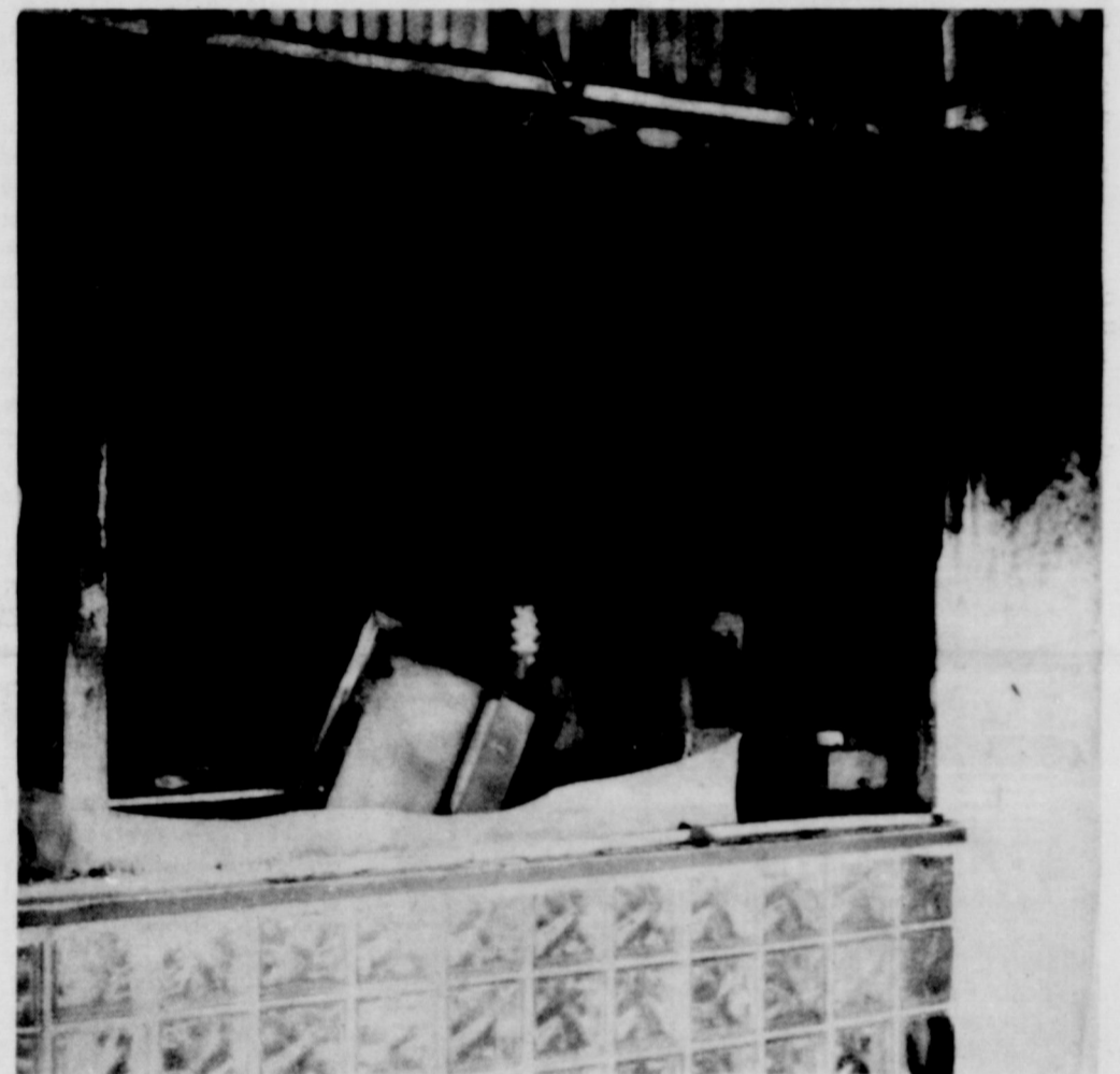
Pictured above is what is left of the Dairy Treat which is located on west main. The fire that ripped through the building around 9:00 Monday night left just the shell of the building. Unknown estimations of damage or origina of fire had been made by Wednesday morning.
