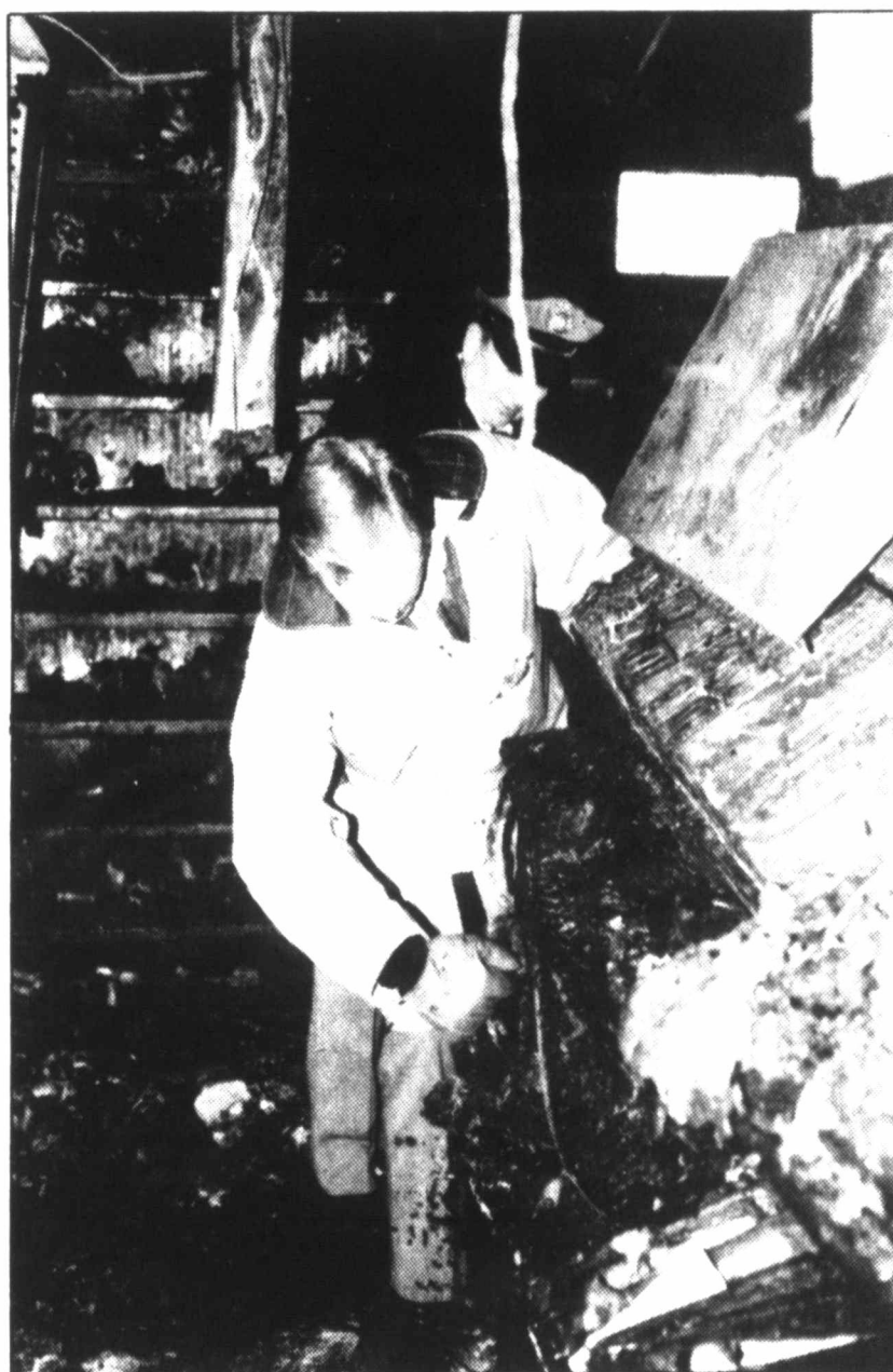
CHARRED REMAINS - Arson investigator Tom Leggett and Assistant Fire Marshall Floyd Steele (in background) sift through some of the charred inventory at Pampa Parts and Supply on W. Brown. (Staff photo by Ed Copeland)
