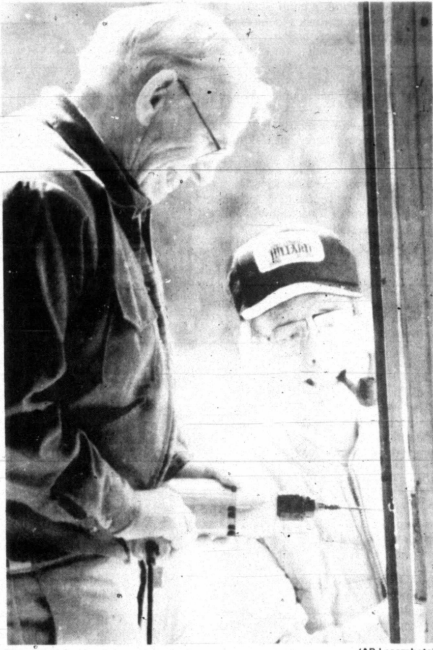
Ken Wilson, left, and Phil Muller, both from First Presbyterian Church of Fort Worth, anchor a door frame in the Ruby Chapel Community Church in Olney.
