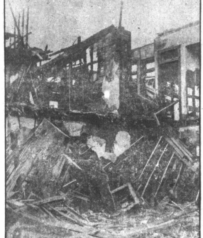
Three persons are known to have been killed and 20 were injured when a fire-ruined building in which they were salvaging unburned wood for fuel collapsed at Homestead, Pa. The picture shows the search for bodies.
