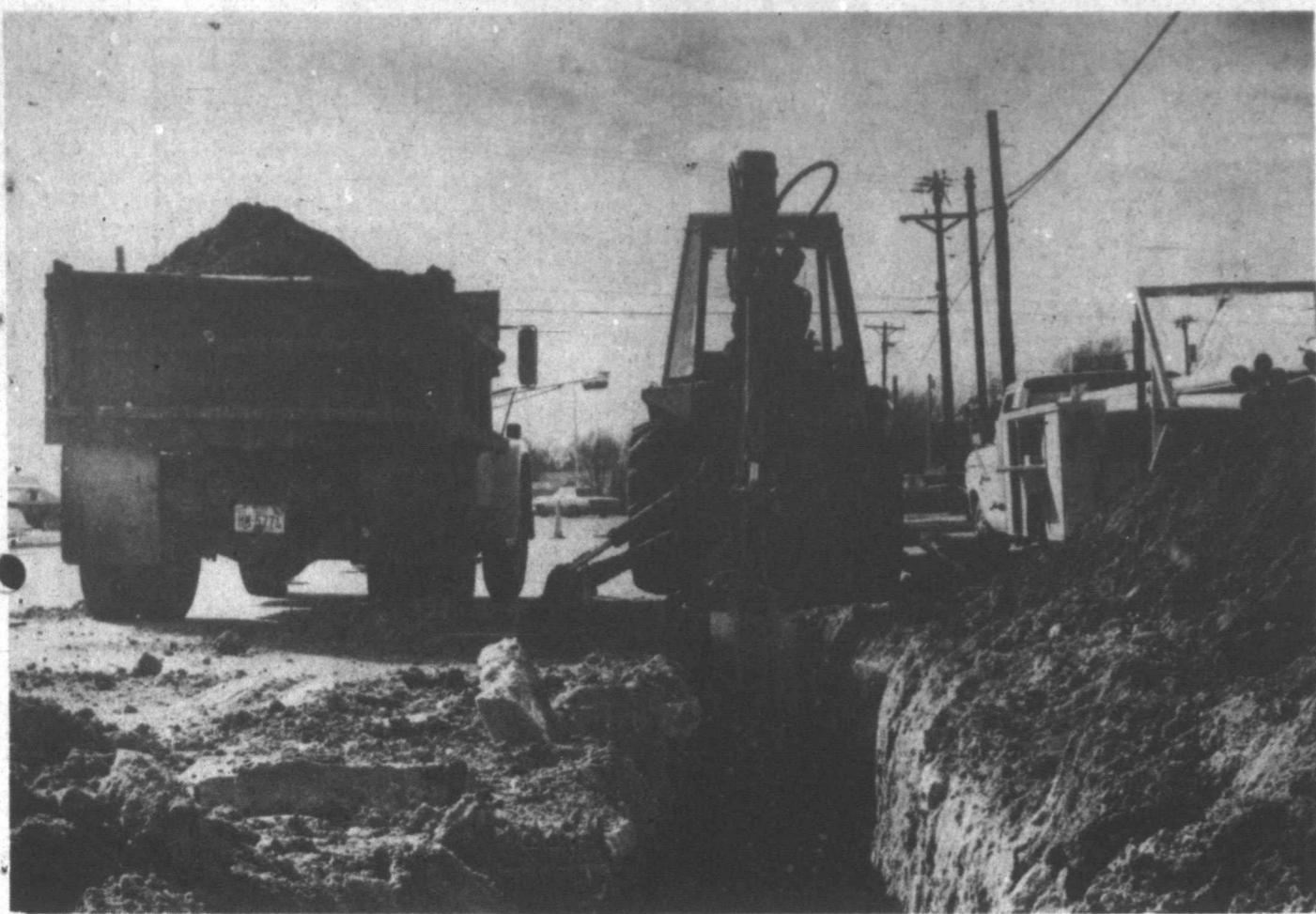
WORKMEN operating what seems to be a mechanical monster repair the corner of Ballard and Browning this week after telephone cables were replaced by Southwestern Bell.
