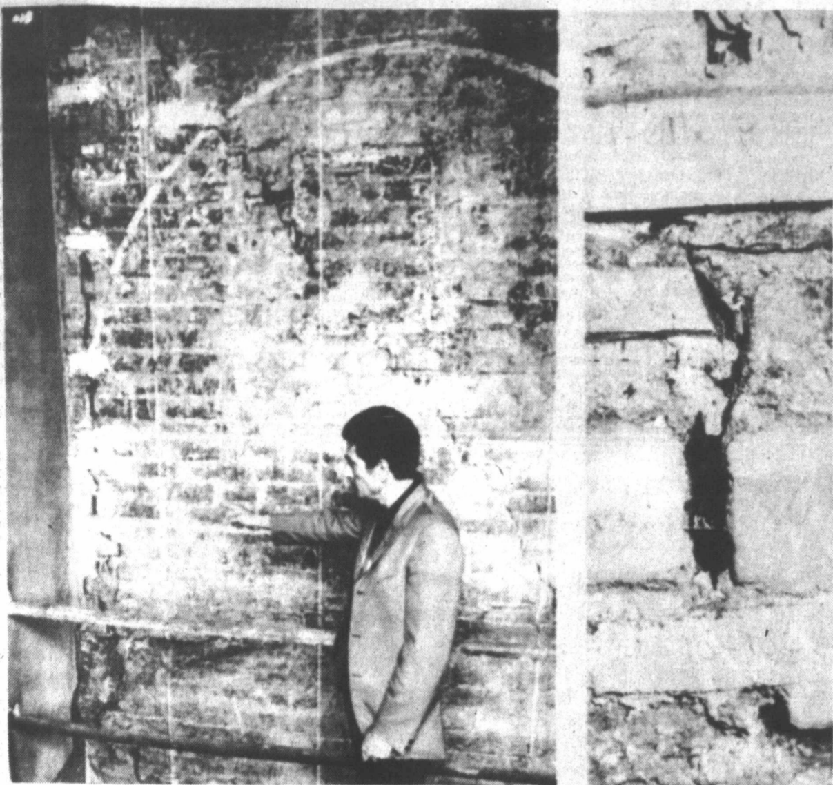
AN ART OFFICIAL points out the large crack which opened on the rear or the wall on which Leonardo Da Vinci painted the famous Last Supper fresco in Milan's Santa Maria Delle Grazie Church. In the picture at right is a closeup of a broken "glass spy" that signalled the fissure slightly appearing on the right border of the masterpiece. (AP Laser photo)
