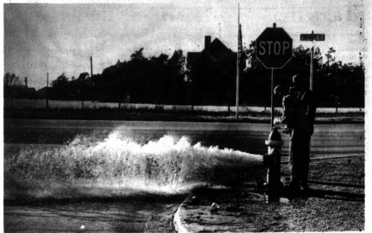
HIGH TEMPERATURES AFFECT CITY EMPLOYEES? With temperatures Wednesday soaring to 55 degrees did these city employees intend to cool off? No, just an average day for Royce Henderson, (checked shirt), and Alton Flowers, (dark jacket) as they release pressure on a water main at Hobart and Kingsmill before making hydrant repairs.
