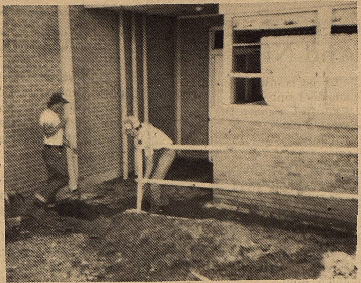
Borden County school employees, Bob Dover and Cam Stone shovel debris away from north doors of the school building.
