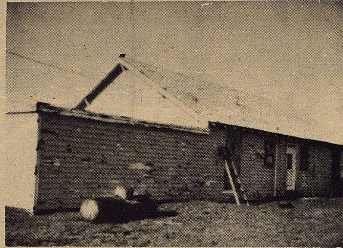
Results of the hail storm can be seen all over town. The north side of this house suffered severe damage as the metal siding could not withstand the high force of the hail.
