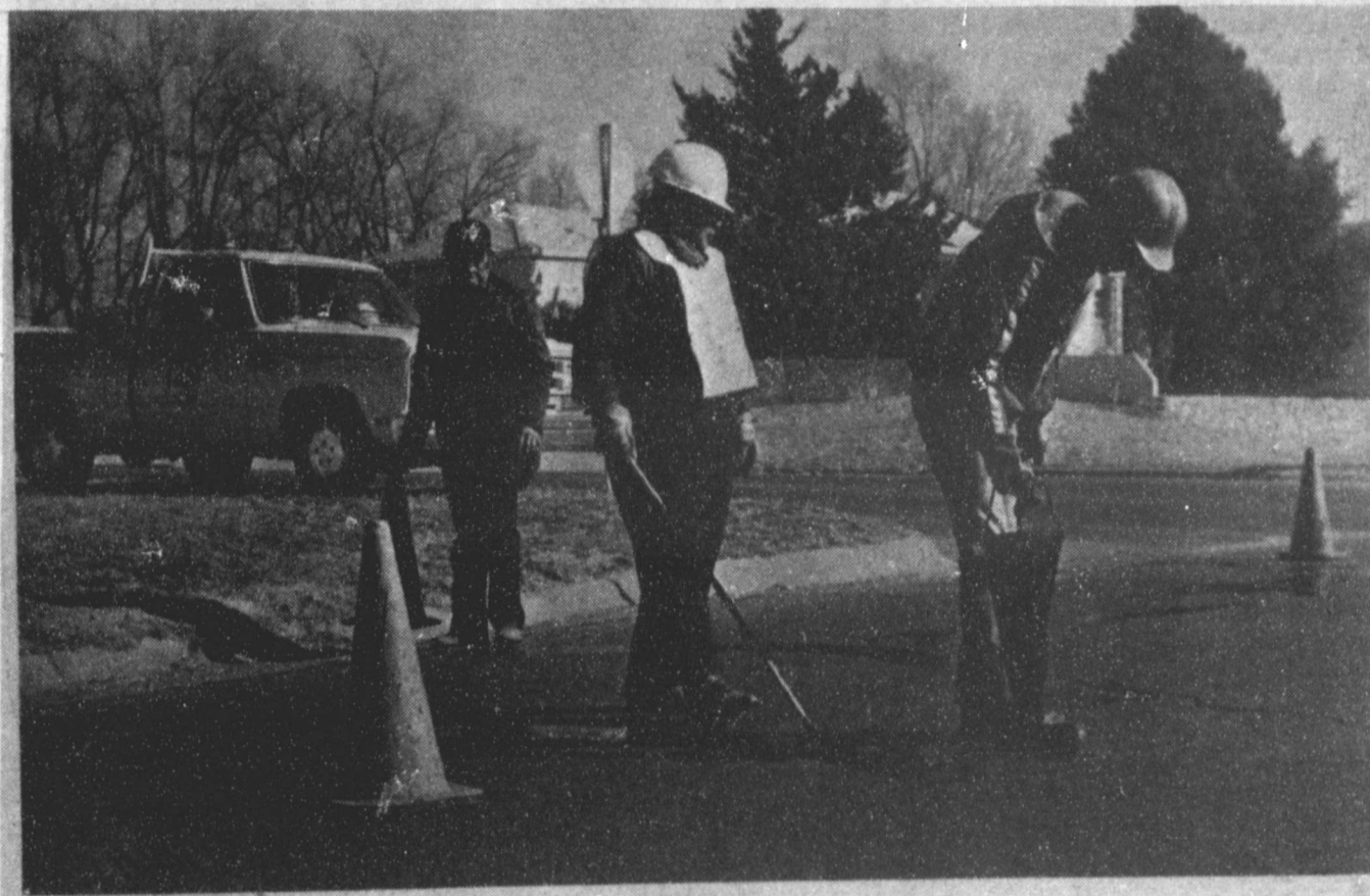
FILLING IN THE CRACKS —Marcos Lopez, background, who is the street superintendent for the City of Muleshoe, is working with his crew as they fill in the 'cracks' in city streets. Also shown in the 'repair process' are Charles Fanning and Bennie Alarcon. Lopez said workmen are taking advantage of the sunny, warm days to take care of the repairs as the nice weather won't last and we can expect some very cold days ahead before springtime.
