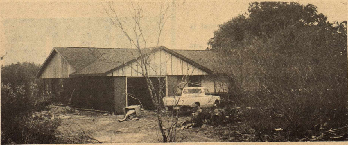
DR. AND MRS. JAMES HARBER ARE CONSTRUCTING THEIR NEW HOME ON FORT CLARK SPRINGS. THIS IS BUT ONE OF NEARLY A DOZEN UNDER CONSTRUCTION AT FORT CLARK AT THE PRESENT TIME.
