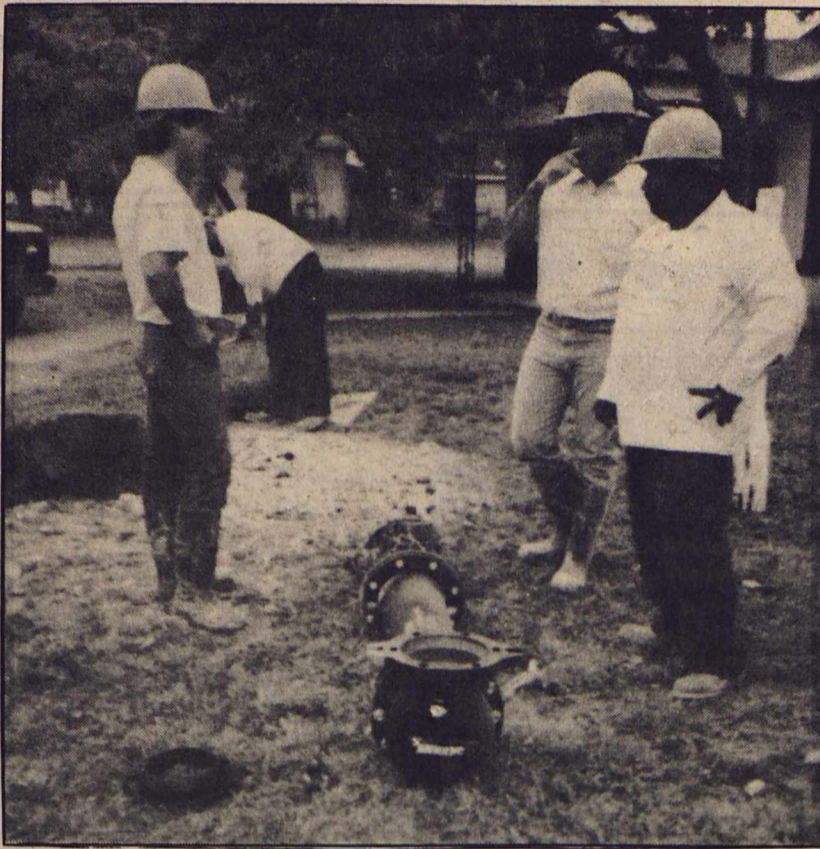
Randy Castilla, Edward Salazar, and Guadalupe "Blue" Sanchez are pictured above about to install new fire hydrant.
