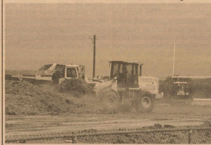
Excitement grows among Coyote players, coaches and fans as crews began construction on the new Borden County turf football field last week.
