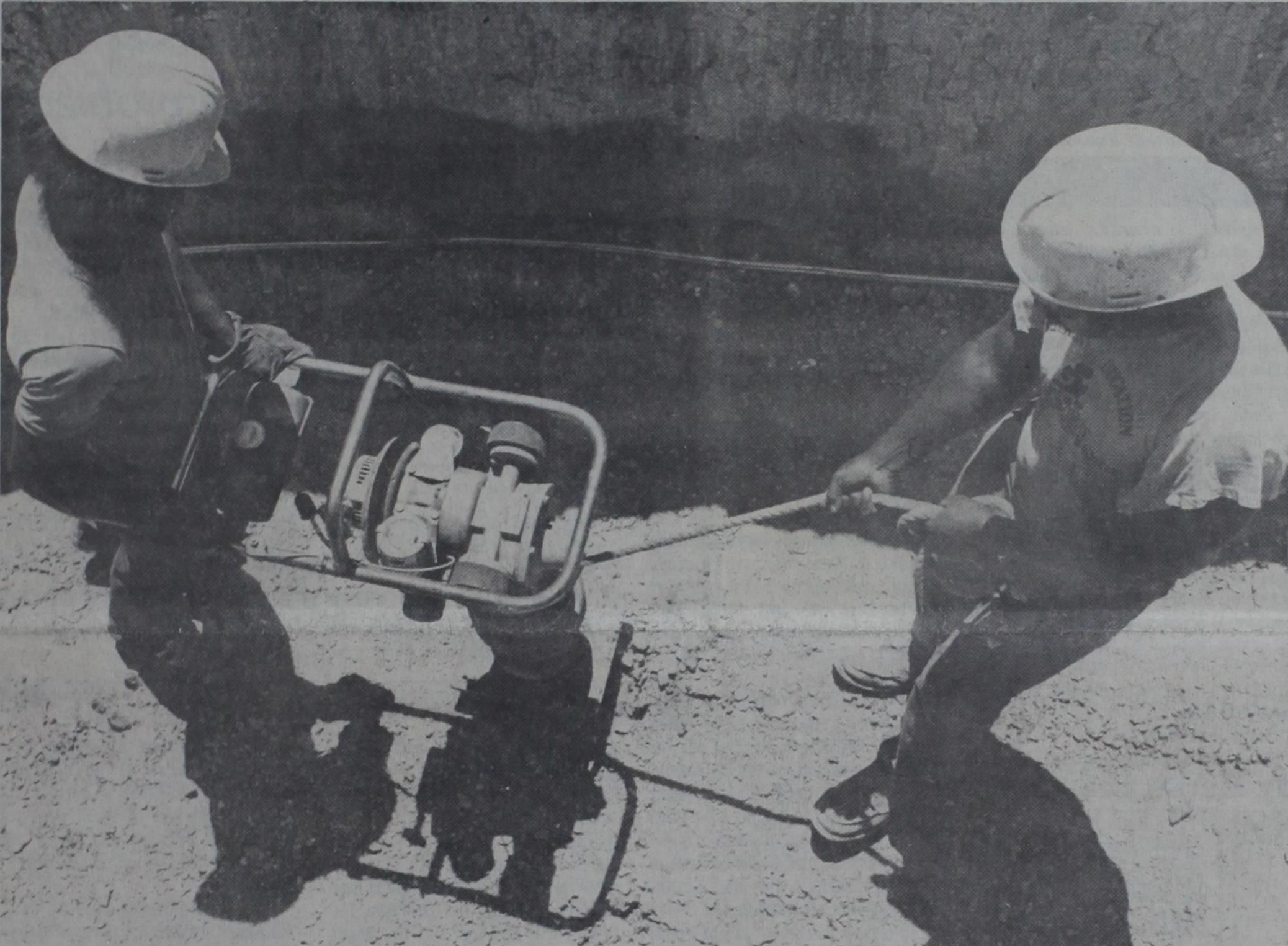
James Adams and Charles Adams, both of Lubbock, pack the dirt around pipes in a ditch at a construction project near the
