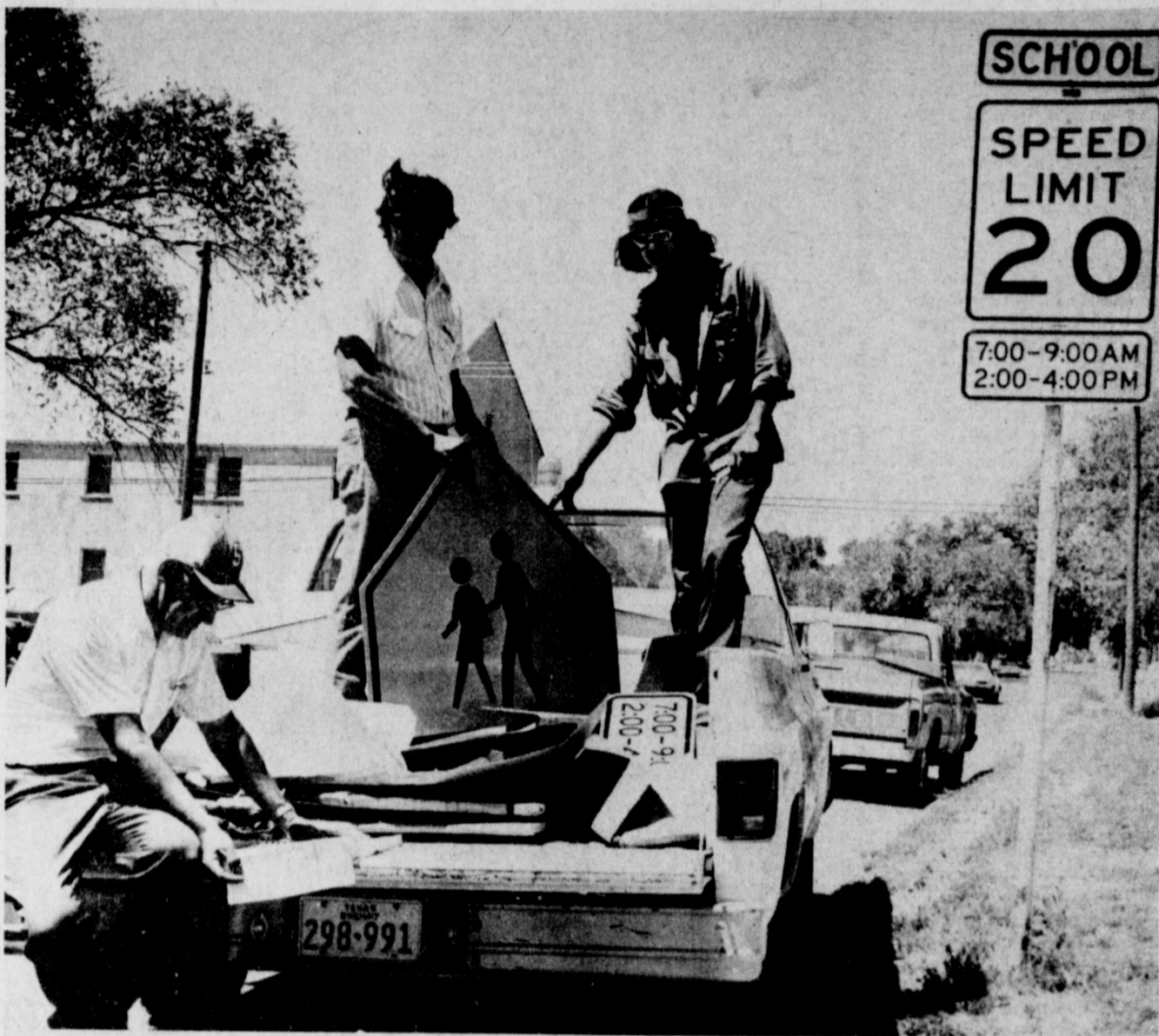
SIGNS OF SAFETY... Muleshoe city workmen are busy this week installing new speed zone signs around all four of the local schools. They also installed signs designating school crossings. City Police Chief Johnny Richards said no warnings will be given persons violating laws in the school zones, but citations will be issued to appear before the judge. Seated is Walter Bartholf, checking for the next place and standing are Marcus Lopez and Johnny Hernandez.
