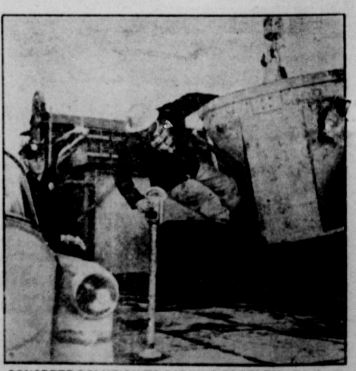
CONCRETE SOLUTION TO PARKING PROBLEM —Construction worker Leo Haynes has the derrick man lower the Officer Ted Horler, left, just as Haynes' parking-meter goes out in Pasco, Wash. Haynes "cemented" relations with the concrete by riding this concrete bucket from atop new City Hall building.
