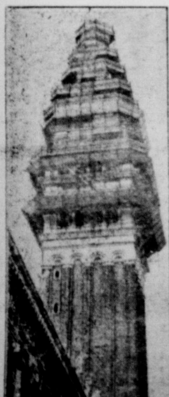
VENETIAN PAGODA — St. Mark's Campanile, in Venice, Italy, assumes the appearance of a pagoda with its temporary ornamentation of scaffolding. The world-famous bell tower in St. Mark's Square is undergoing a parental cleaning of its marble facing.
