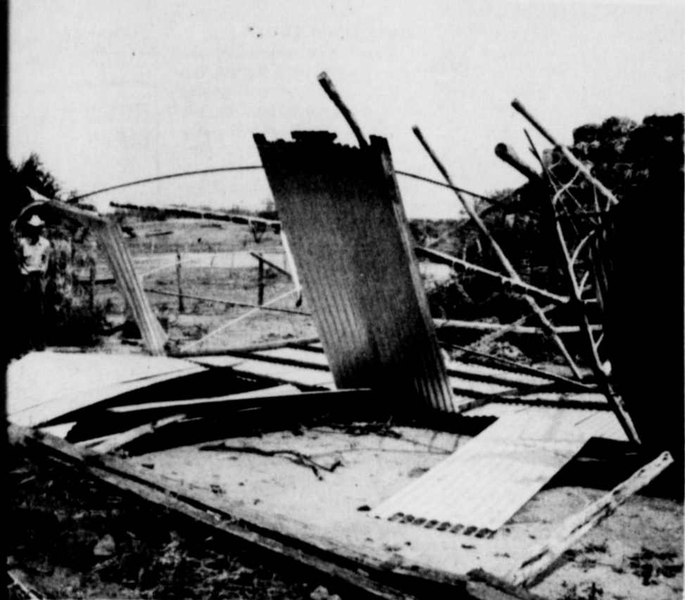
STORM DAMAGE —Jimmy Russell's barn which was destroyed in a tornado Wednesday afternoon of last week.
