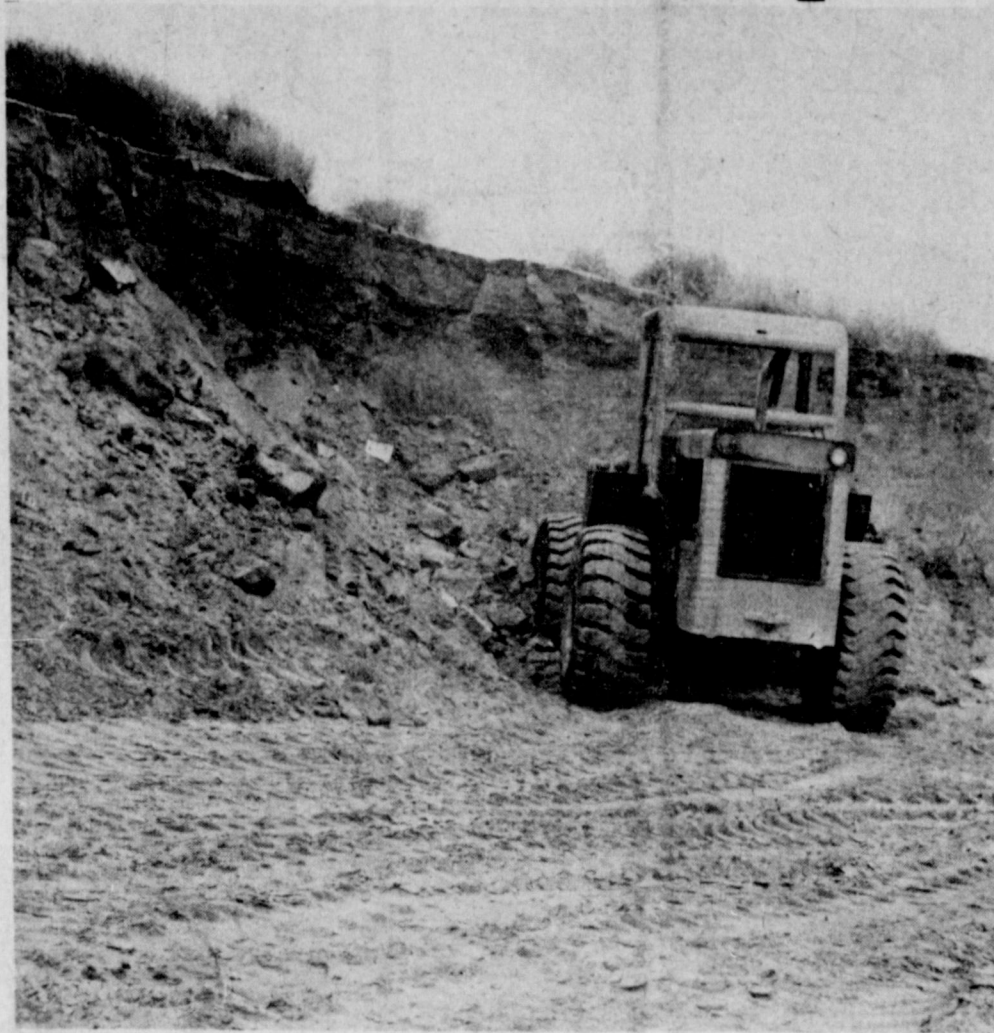
LANDMARK WILL BE MISSING--The sandhills at the city dump will be a thing of the past in a short while. Workmen are busy removing the longtime landmark and are using the soil to fill the site of the labor housing project east of the old city park. Years ago, trees dotted the top of the sandhills and youths parked at night at that location, just above the tractor seen here. Many picnics will be remembered at the trees. Progress has forced the removal of the longtime landmark.
