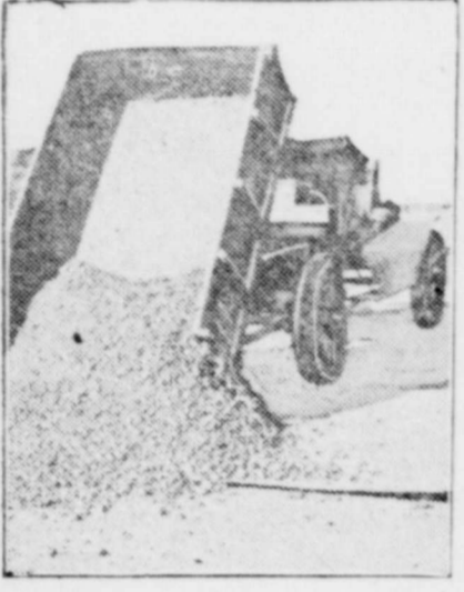
One Type of Road—Truck-Load of Hot Concrete Being Dumped Ready for Surfacing.
