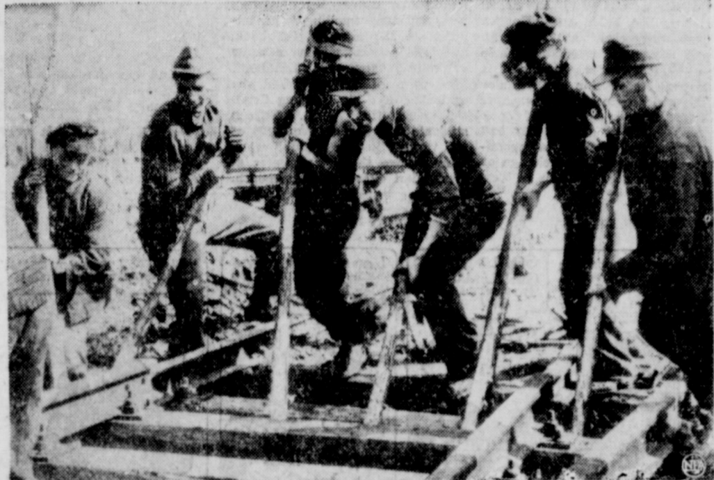
Hope mounts that the Berlin Blockade will be lifted. Here, German railroad workers repair switch-rails at the British sector's Grunewald station, preparing the line for resumption of rail traffic to the Western Zones. (NEA Telephoto.)
