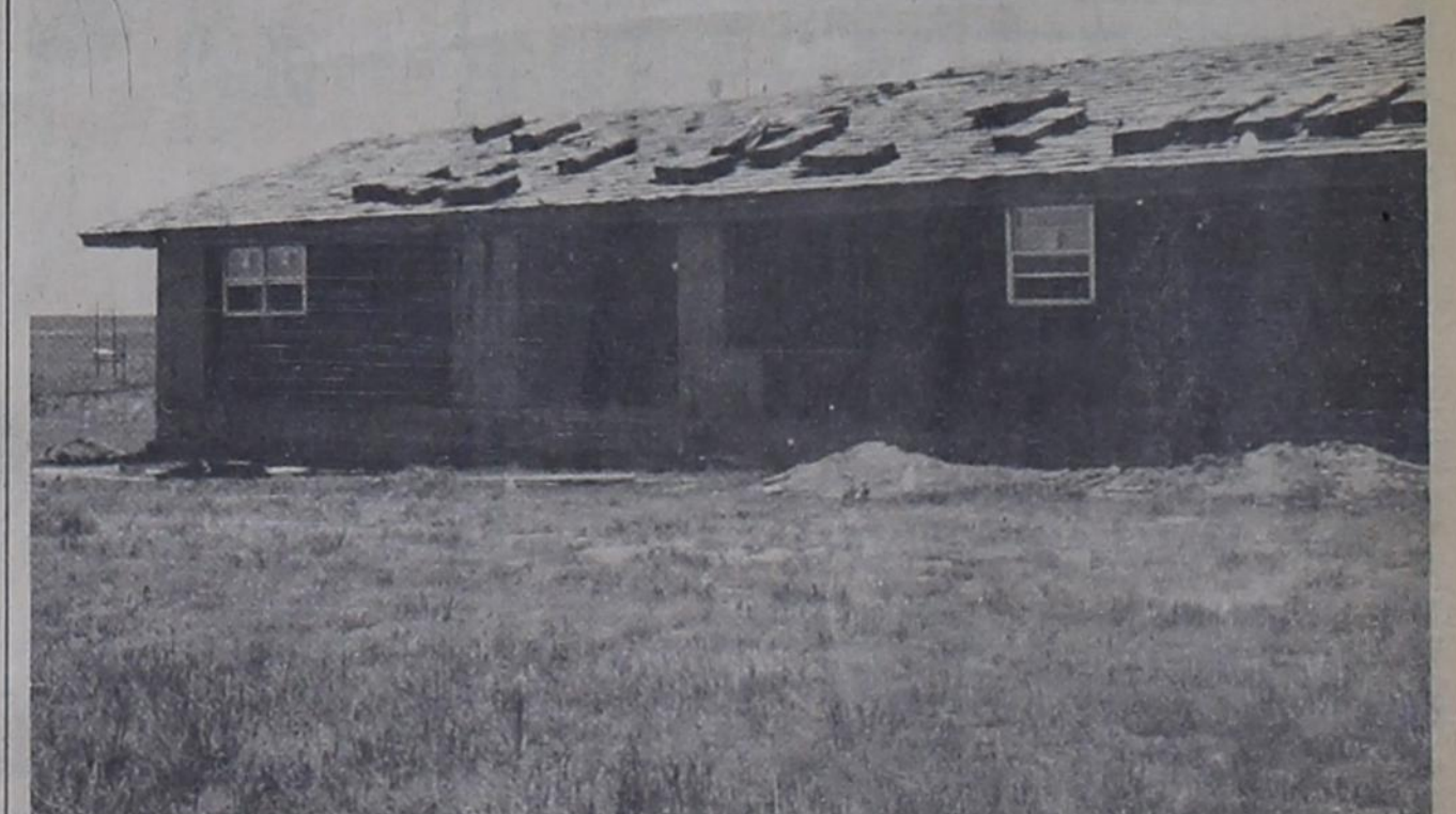
HOME UNDER CONSTRUCTION ...The new four-bedroom, two bath, brick home of Mr. and Mrs. C.E. Trimble is scheduled to be completed July 1. The home is located on FM 1731 next to
