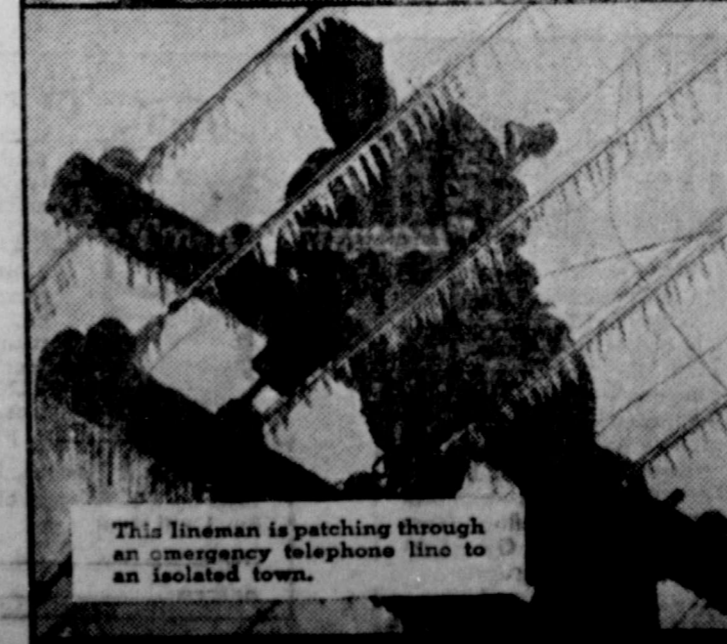
Repair crews, rushed into January sleet storm area, found miles of telephone line flattened by ice.
