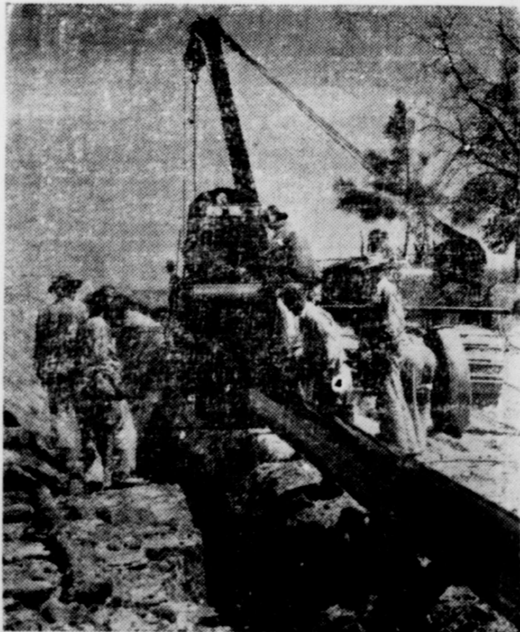
ONE OF SEVERAL NEW PIPELINES recently completed to keep gas service ahead of increasing demand. Since V-J Day, Lone Star has invested over $100 per customer in new facilities to assure each a dependable supply of gas. Yet for a year around average of less than 15c per day, you enjoy carefree heating, silent refrigeration, automatic cooking and abundant hot water supply using Lone Star Gas Service.
