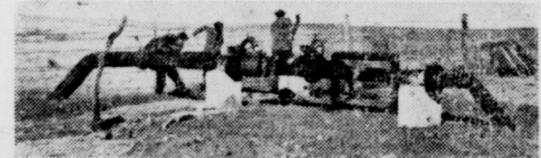
BEHIND YOUR GAS SERVICE there is something to build, paint, or repair every day—oftentimes in remote places. Above, a crew cleans up debris around control valves which are part of a new compressor station.
