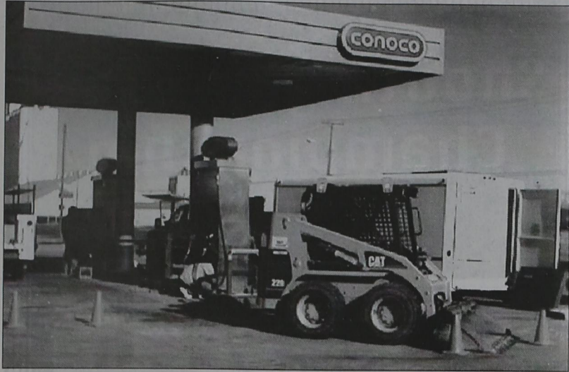
BRAND NEW PUMPS--Bovina's Fast Stop had new gas pumps installed a couple of weeks ago to serve their customers more efficiently.
