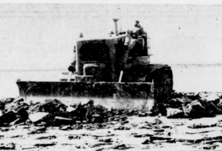
SECOND STEP — After the bulldozer has plowed up the flightline with a steel fork which is a part of the multi-ton piece of equipment, the scooping of the flightline begins. Construction started Feb. 1. (AIR FORCE PHOTO)
