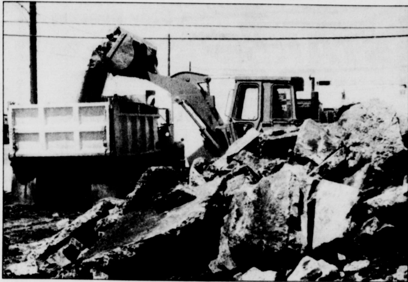
The city was busy working on the site of the new City Hall this week. City employees removed an existing foundation and hauled it away. After the lot has been leveled, a new foundation will be poured. (Staff photo)
