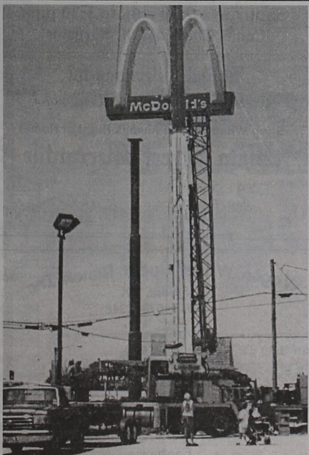
There was quite a bit of local interest last Friday afternoon when the new McDonald's sign fell into place. Located at the corner of Broadway and Main, the new store is scheduled to open its doors today (Thursday) with a grand opening on Friday. The restaurant will open under the direction of franchisee Bill Cohen of Levelland, who has owned and operated the McDonald's in that community since 1995. Its opening will create a number of new jobs in Post. (Photo by Thomas Zachary)
