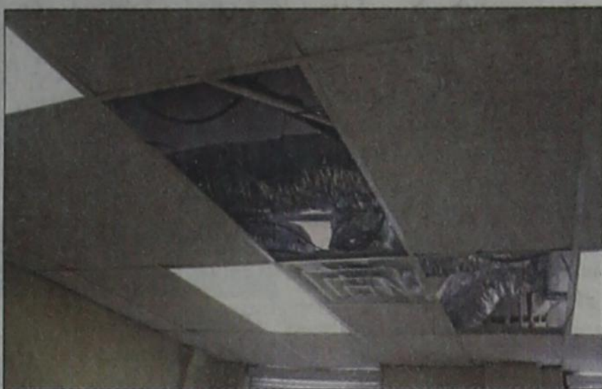
Work continues for installing central air in the courthouse. Pictured is the ceiling of Garza County Clerk Jim Plummer. This will replace the old and noisy window units that have been used in the past. Work is expected to be completed soon.
