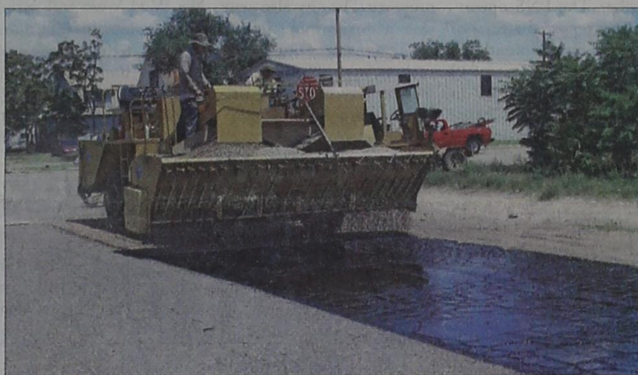
Streets in the city have been getting a new covering this week as 14 blocks were sealed with a new cover of tar and rock, otherwise known as chip seal. The neighborhood east of the railroad tracks of Henry, Jasper and Oak streets along with 6th, 7th, 10th, 11th, 12th, and 13th were coated and sealed to the tune of just under $100,000, which was the budget limit for the project. According to the city, similar projects will be explored each year for the same amount of money until all the streets are re-sealed. After that, the streets will be put on a rotation project as per need and available funds for future projects.
