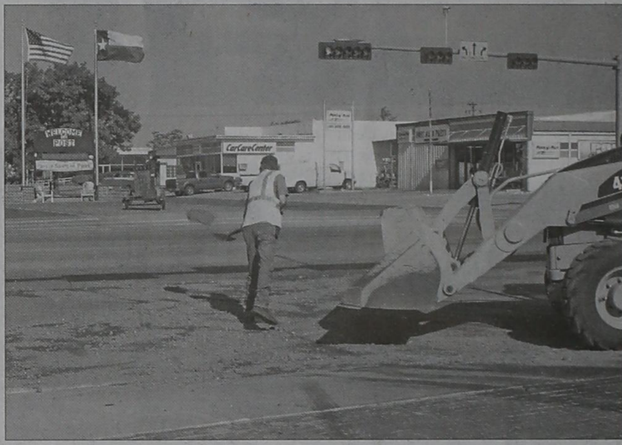
A City of Post employee spreads dirt on a fuel spill Friday morning at the intersection of Main St and Broadway. It is presumed that a truck carrying the fuel unknowingly spilled the fuel while turning the corner. The incident happened right in front of City Hall and was quickly handled.
