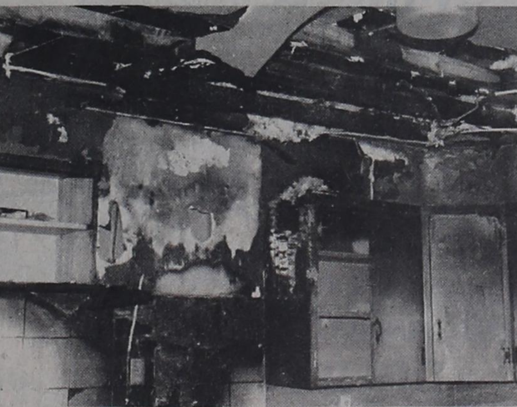
EXPLOSION RESULTED.... Shown are the ceilings and cabinets destroyed in last week's fire at the home of Eddie Don Lide, 401 Avenue E. The fire was caused when a utility pole was blown against the gas meter at the home, causing a heavy flow of gas into the cook stove. The stove exploded with the gas reached the pilot light. No one was home at the time of the fire.
