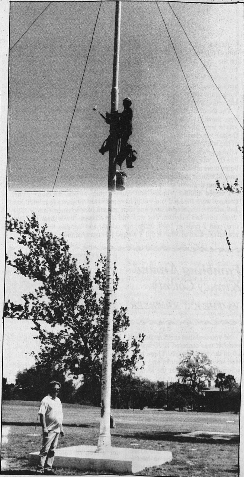
Monday, April 17, 1995, the flag pole on the Parade Ground was being repainted. The pole is about 85 feet tall and at this point the painter was about 30 feet from the ground.
