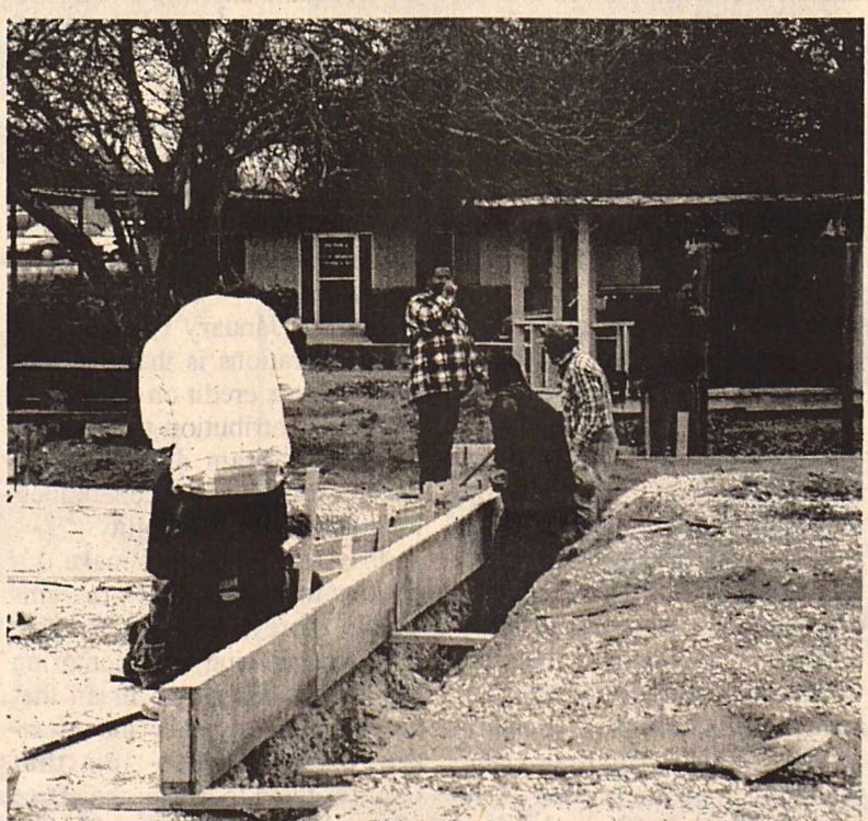
Pictured above are construction workers from Prieto & Sons Construction Company laying the forms and digging the footings for the foundation of the new EMS building.
