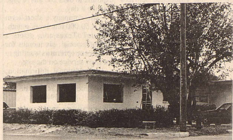
Work is progressing rapidly on the Kinney County United Medical Center's new pharmacy. A spokeswoman said Wednesday that it is hoped the new building will be ready for the pharmacist to move into next Tuesday.
