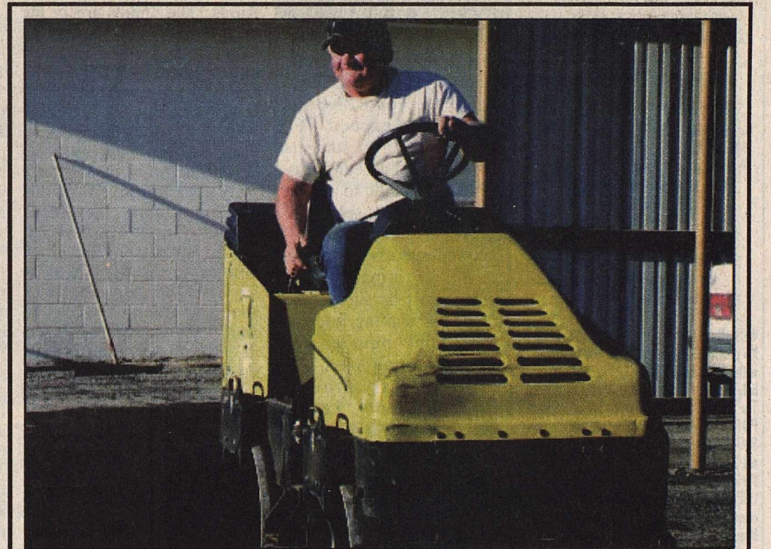
Black Top Man Kenneth Everett of Kenneth Everett & Sons from Pleasanton repair the parking lot at the Brackettville United Medical Center.
