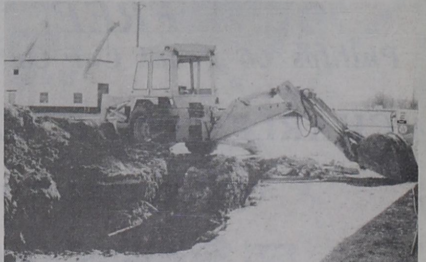
TANKS REPLACED.... Wieland Tank and Environmental Service of Clovis, New Mexico, began work at the Texaco Station located on Highway 60. Work began Monday, November 18 and, according to owner/operator Paul Jones, should be completed by Saturday, November 23. The tanks will be replaced with above the ground steel tanks.
