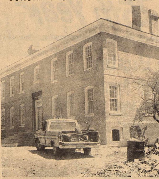
The James Hunt family residence is under construction. The large brick home is located on Sonora Drive near the newly constructed La Casita Apartments.
