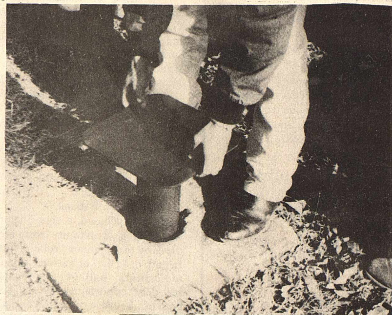
CAPPING THE WELL - The local FFA Chapter is working in cooperation with the local water district to construct these metal caps to be used in abandoned wells found in the city and county. If you know of any abandoned wells please contact Mike Smith at the local water district office, 201 E. Main, Suite 101 or call 387-2369.
