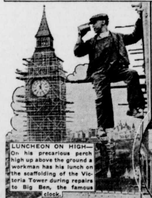
LUNCHEON ON HIGH —On his precarious perch high up above the ground a workman has his lunch on the scaffolding of the Victoria Tower during repairs to Big Ben, the famous clock.
