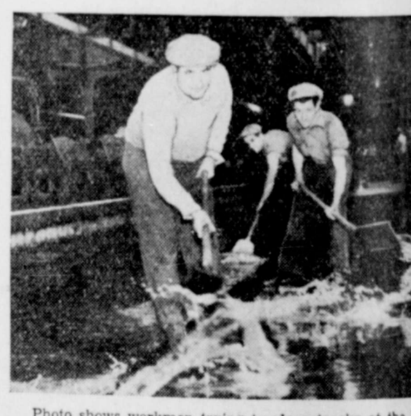
Photo shows workmen trying to clear tracks at the Union Station in Chicago of a flood estimated at three to ten feet deep. A 30-inch main burst putting 14 railroad tracks out of commission. The also flooded portions of the new post office. Passengers and urban trains were forced to alight from inbound trains about a mile from the station. Damage was estimated at $200,000.
