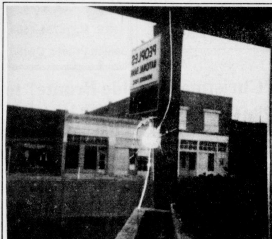
REFLECTIONS — No matter how you look at it, this softball-size hole in the plate glass window at Peoples National Bank is costly. Vandals broke windows in five other downtown businesses early last Friday morning.
